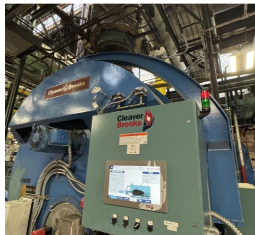
Upgraded Boiler Control Panel
