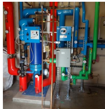
Typical New Instantaneous Water Heater
